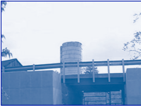
Dans Run Slab Bridge - An example of a bridge with FRP rebar
