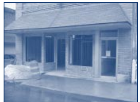
Picture taken 9/20/01 showing completed concrete work and reframing of Dr. Barit's office.
