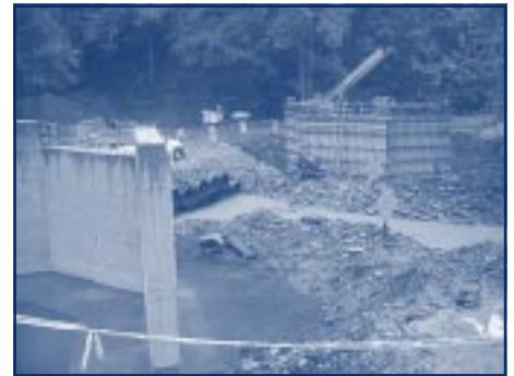
Progress is being made on replacing the Davis Street Bridge crossing Slab Fork Creek, near the caution light in West Mullens.
