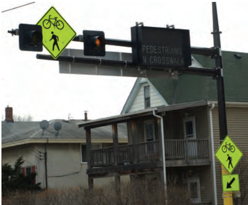
OVERHEAD FLASHING SIGNAL BEACONS
