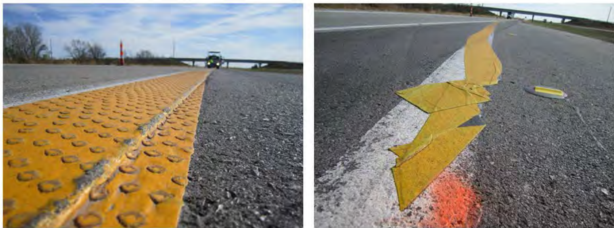
Figure 6. Pavement Marking Damage in a Work Zone
