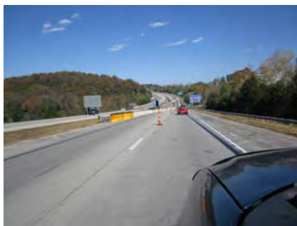
Figure 15. Example of Disallowed Black Paint Covering Temporary Pavement Markings (Source: Leidos)
