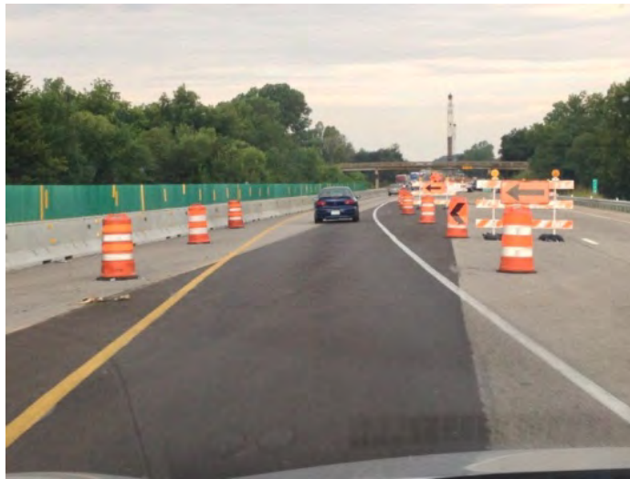
Figure 5. Use of Paint on Lane Shift on I-44 in Oklahoma. (Source: Leidos)
