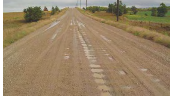
Figure 61. Photo. Too little crown (<4%).
