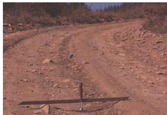
Figure 2. Photo. Poor unpaved road.
