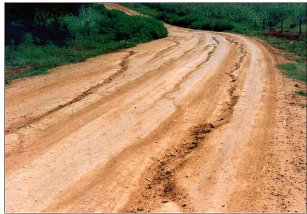
Figure 37. Photo. Longitudinal erosion.
