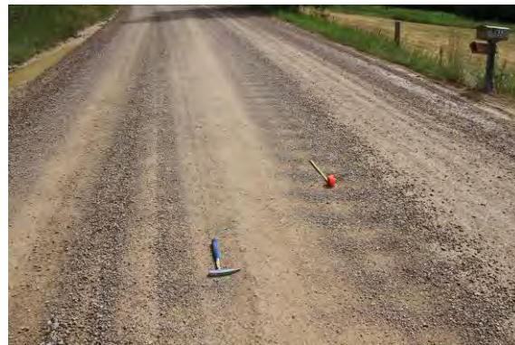
Figure 59. Photo. Chloride applied to poorly prepared road.
