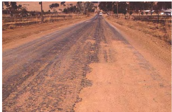
Figure 17. Photo. Broken crust.
