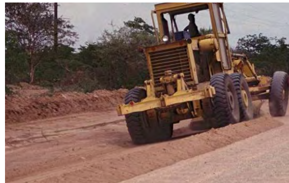
Figure 62. Photo. Too much crown (>6%).
