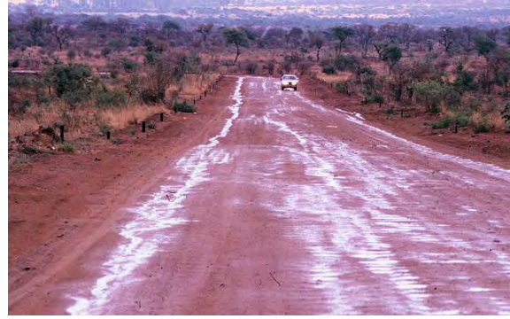
Figure 15. Photo. Excess runoff of chemical treatment.
