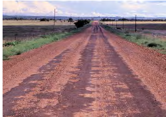
Figure 70. Photo. Insufficient additive application.
