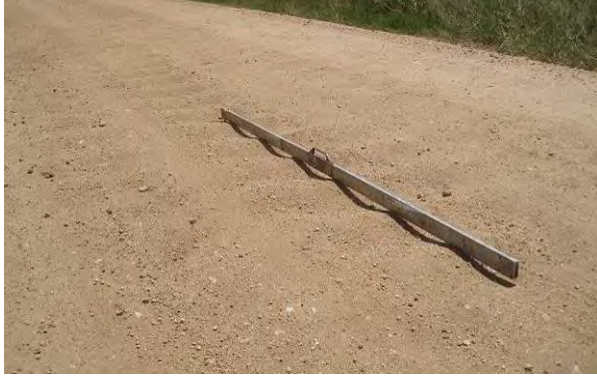
Figure 38. Photo. Washboarding (corrugation).
