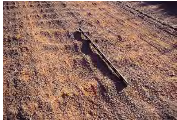
Figure 58. Photo. Poor gravel selection for treated road.
