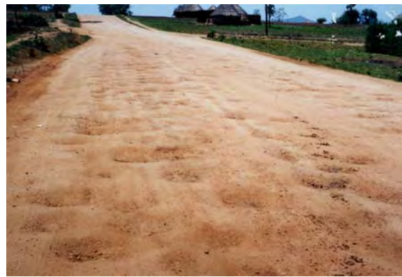
Figure 23. Photo. Potholes caused by poor drainage.
