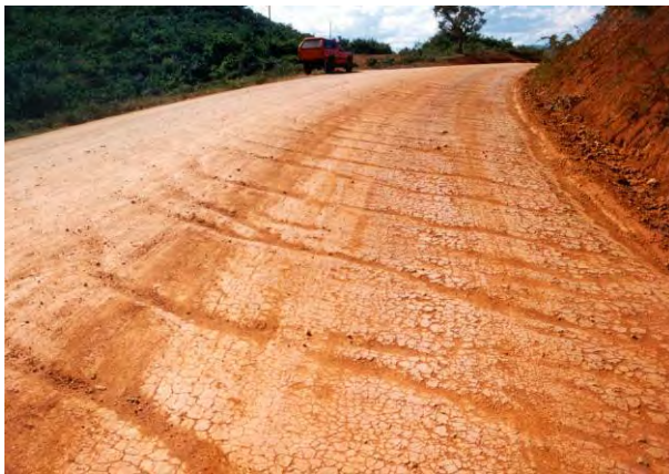
Figure 36. Photo. Transverse erosion.
