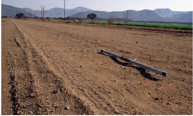
Figure 39. Photo. Washboarding and raveling.
