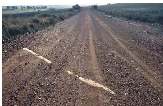
Figure 20. Photo. Insufficient, poor quality gravel.
