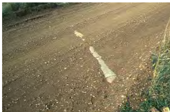
Figure 26. Photo. Road requires upgrade before treatment.
