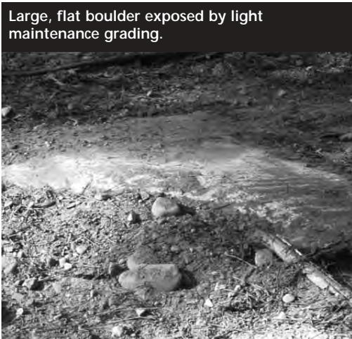
Small rocks create potholes and become a travel hazard.
