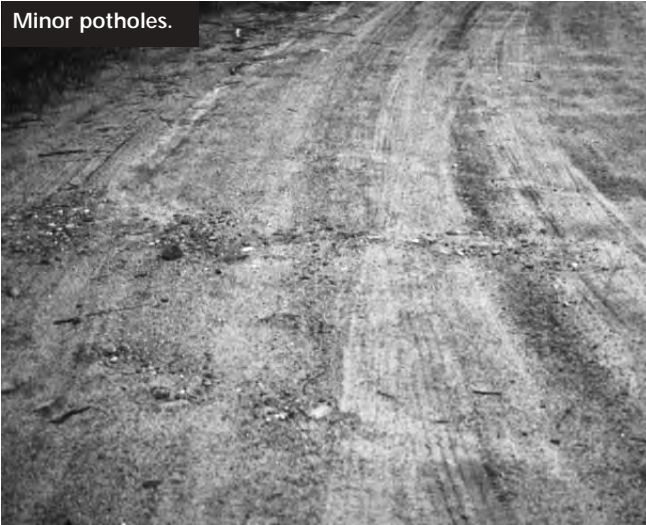
No grading, crown or ditching leads to severe potholes.
