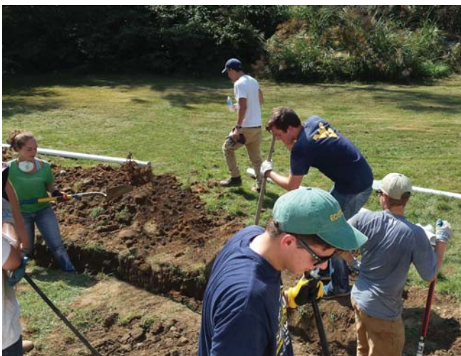
These student volunteers are working on digging a trench that is a necessary part of the process for getting the family's home connected to their septic tank.
