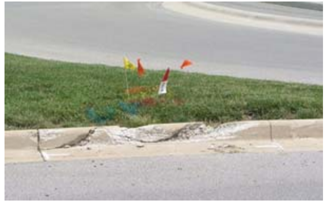
Figure 2. Example of damage to the curb in a roundabout from a plow.
