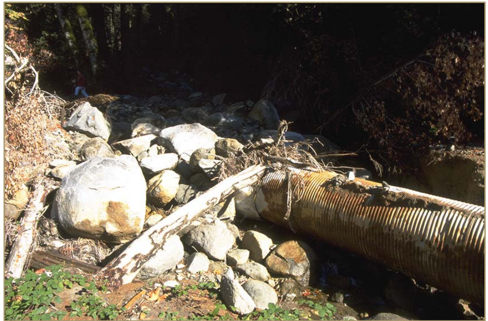
This photo by Gordon Keller depicts a plugged culvert that failed.
