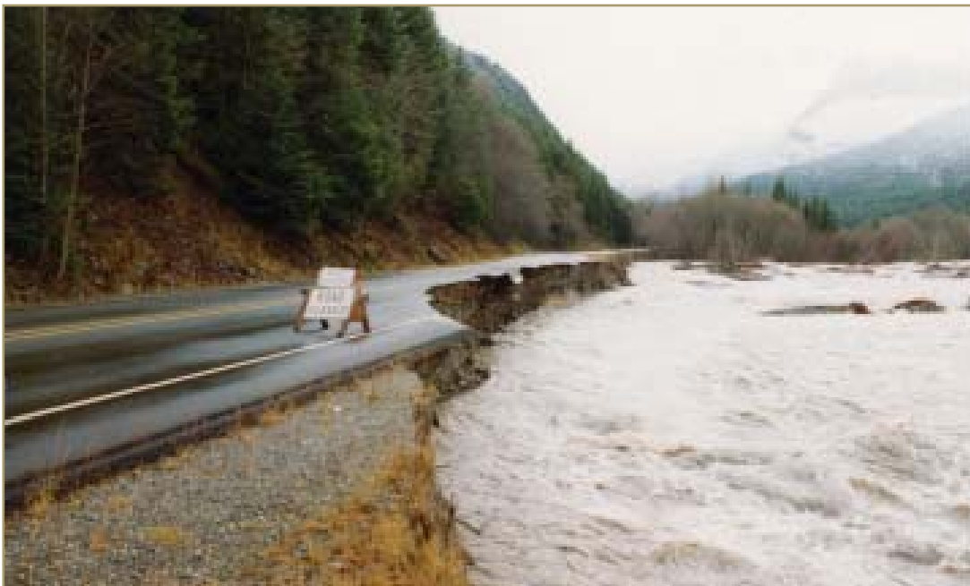
Extreme weather events may cause roads to wash out. Photo taken by Gary Ketcheson.
