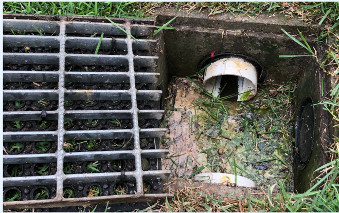
Photo by Canva - Catch basin with a sump collecting grass.
