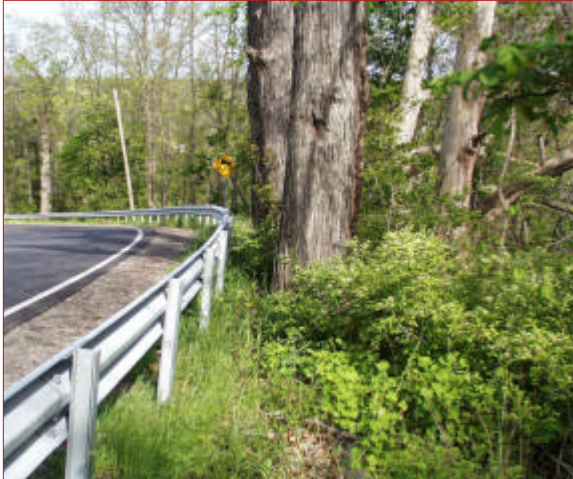
Figure 1: This rail does not have enough deflection distance to protect traffic from the tree
