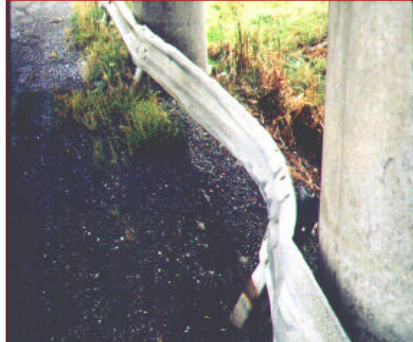
Figure 2: This rail deflected into the concrete bridge column and failed to protect the people in the car
