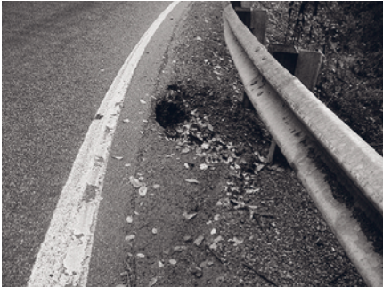
Shoulder conditions such as this shoulder washout are typical safety concerns being found.
