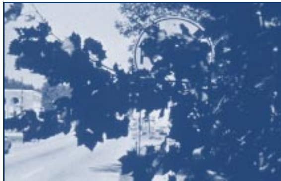
This Railroad Crossing Warning sign is blocked by foliage. The lack of visibility could cause a motorist to miss seeing this sign and contribute to a possible accident. The foliage should be cut as soon as possible. photo from T2 file
